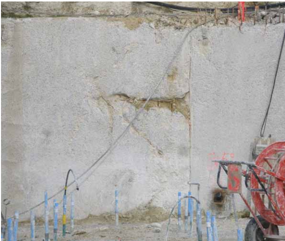
FIGURE E.2: Examples of inclusions of a diaphragm wall and a pile [pile photo taken from Figure 9.14b, FHWA GEC10]
