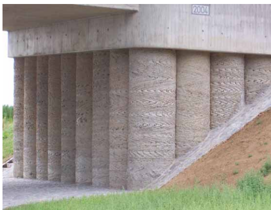
FIGURE E.1: Examples for piles with grooves, not affecting the minimum cover for durability
