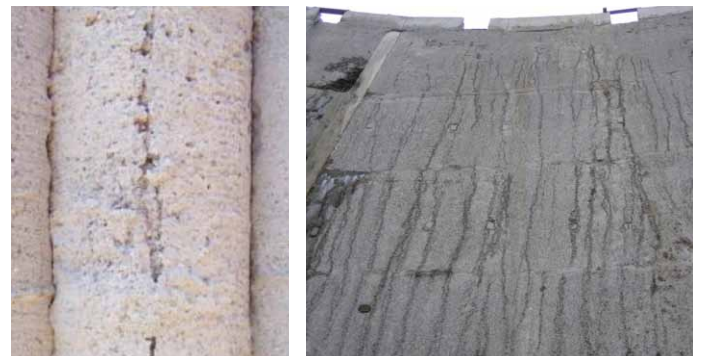
FIGURE E.3: Examples of channels running up the surface of a pile and a diaphragm wall
